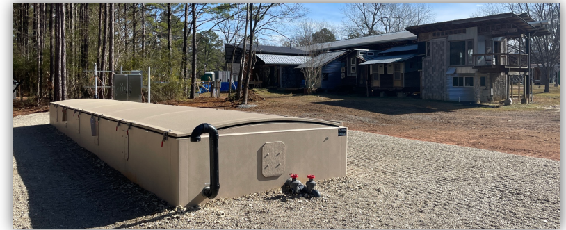
Decentralized system installed in Newbern, AL
